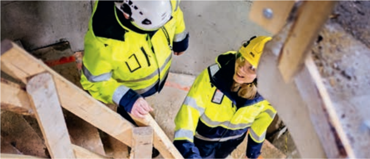
A challenge for Assemblin is that our clients apply different safety requirements. We have therefore introduced our own minimum standard for personal protective equipment at construction sites, which applies regardless of our clients' requirements.
